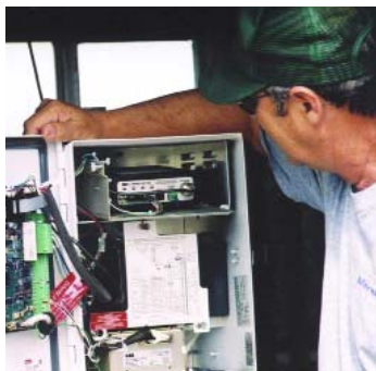
PNR Lead Instrumentation & Electronics Tech Bob Carroll demonstrates the MDS 9710 transceiver installed inside an ABB TotalFlow Flowmeter at the Ulysses Production Facility.
